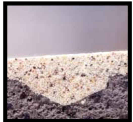
Cross-sectional view of ET-2000 process combined with EF-1988 and spray applied to deteriorated concrete (with hand trowel finish).
