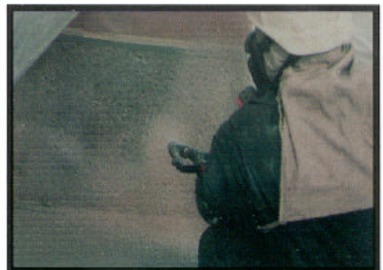
Secondary containment for acid products. Sand/fiber fillers injected into ECOSYSTEM ® expanded materials and applied direct-to-concrete.
