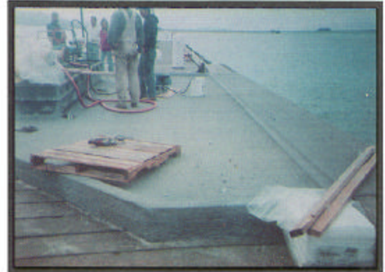
Wood dock secondary containment. Sand/Fiber fillers injected into ECOSYSTEM ® expanded materials for heavy physical abuse. View 3 hours after application.
