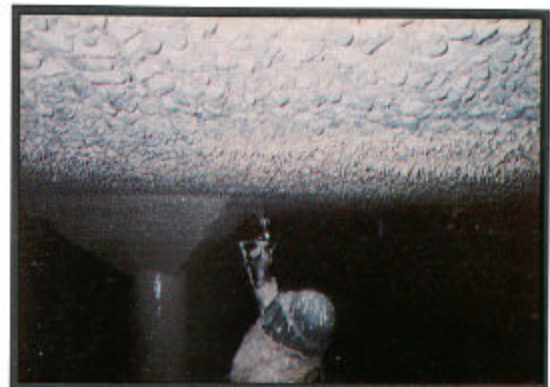
ECOSYSTEM ® expanded materials applied direct to severely degraded concrete in sewer treatment clarifier.
